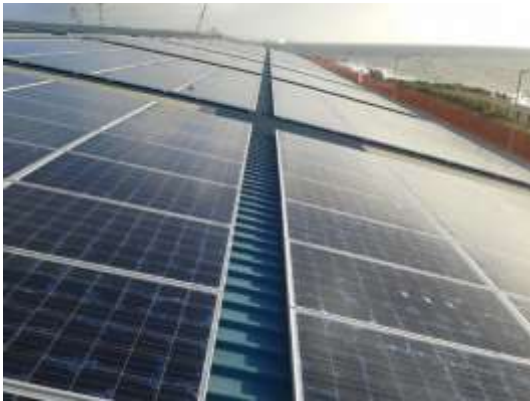
Solar panels on warehouse roofs
